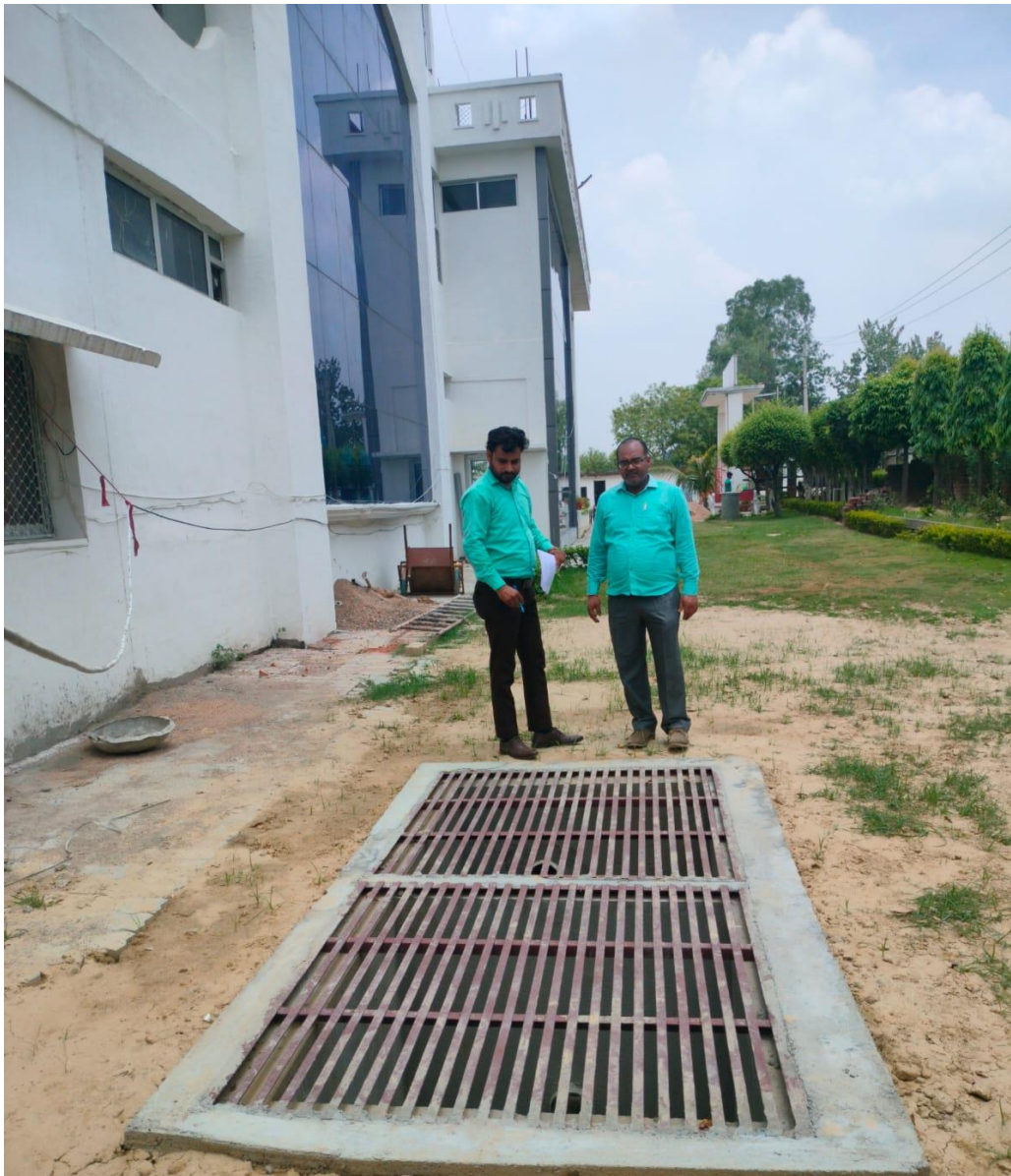
Photograph showing the Rain Water Recharge Structure / Pit in Campus Area
